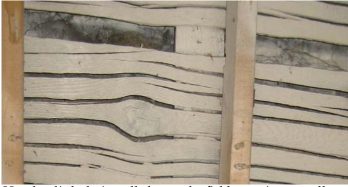
Hand-split lath, installed over the fieldstone inner walls (2x4s added later as the structure for apartment walls)
