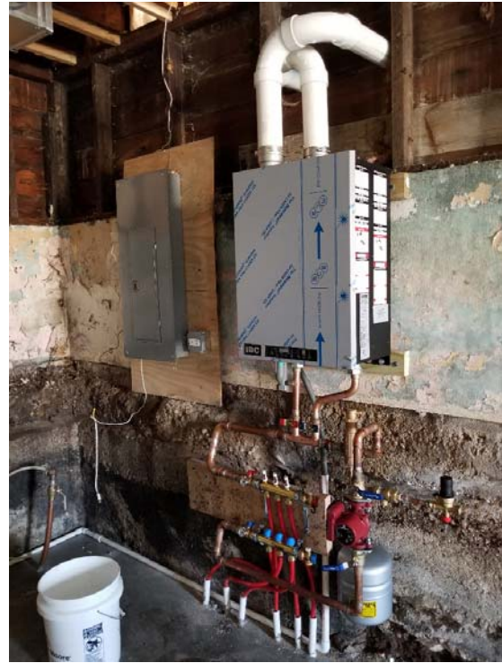
Boiler for concrete floor radiant heating system
