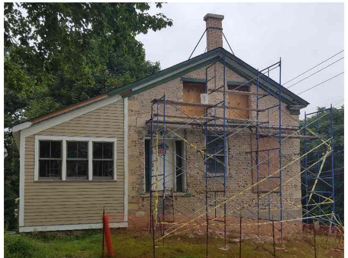
Scaffolding in preparation for repairing the front facade of the Nancy Kimball Cobblestone House on W. Chicago St.
