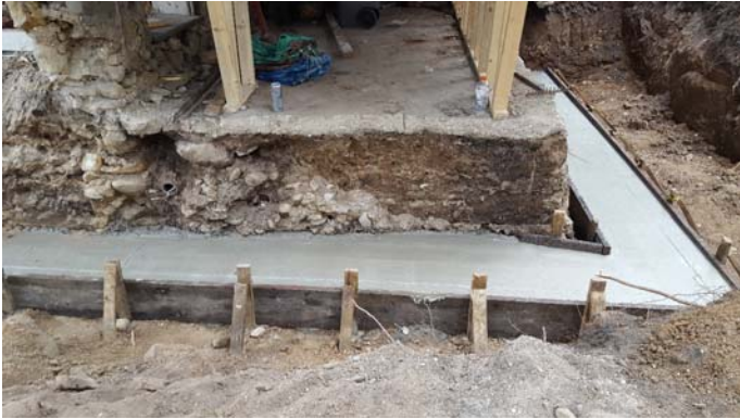
New concrete footing for north wall, to provide adequate support for the slumping wall torn down and soon to be rebuilt
